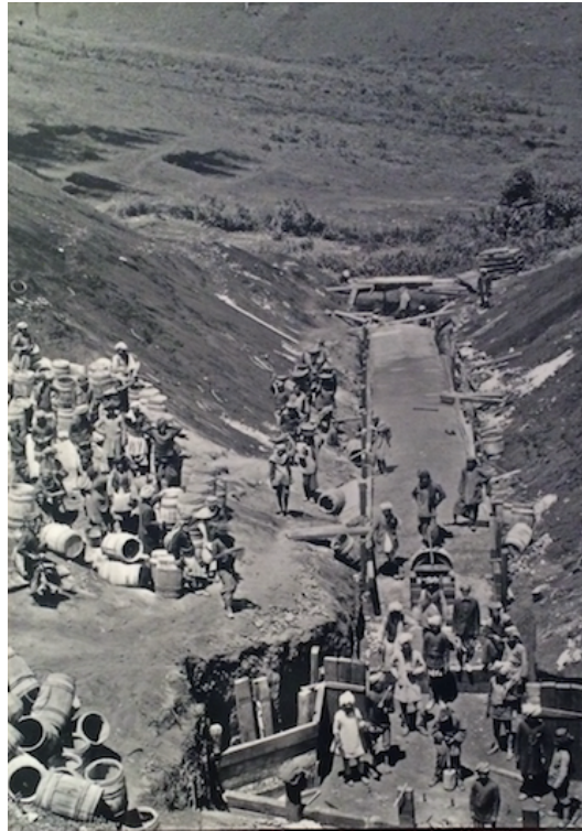
Constructing the Uganda Railway in British East Africa, culvert at mile 348 National Museums of Kenya
